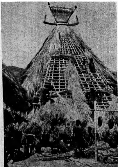
Thatching the roof of a large lineage house. Note the gongs, which are played at intervals during the course of the work.
